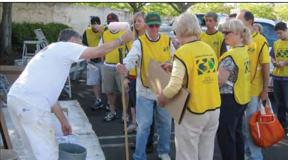
Mike Simpson, from Glidden Professional, handed out paint and formed groups to paint retaining walls along the 241 Tollroad from Rancho to Las Flores. PHOTO BY JOLENE BASS
